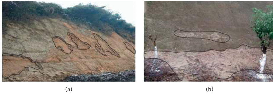
FIGURE 1: Spalling of the shallow surface of slopes in the intermittently frozen area. (a) Flaky exfoliation. (b) Fragmentary exfoliation.
