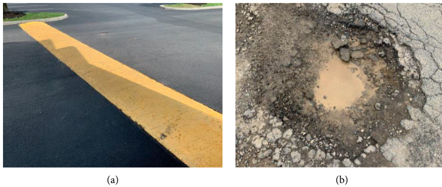
FIGURE 12: Pavement deterioration samples in Blacksburg, VA. (a) Speedbump sample. (b) Pothole sample.
