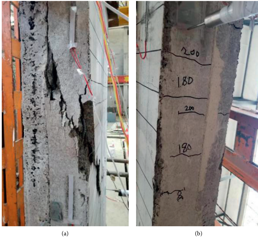
FIGURE 12: The experimental phenomena: (a) the damage of the middle column; (b) the cracks at the top of the hole.
