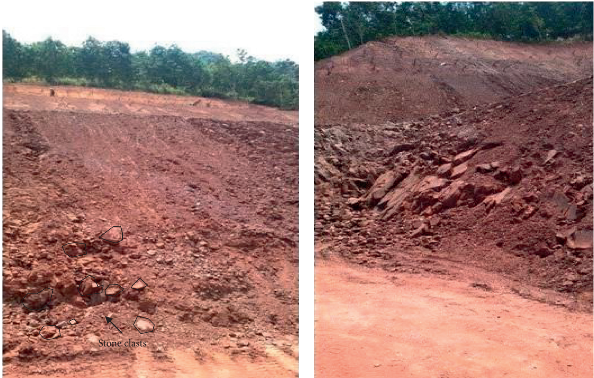
FIGURE 1: Surface of the highway slope along XiaoMo highway in Yunnan Province.
