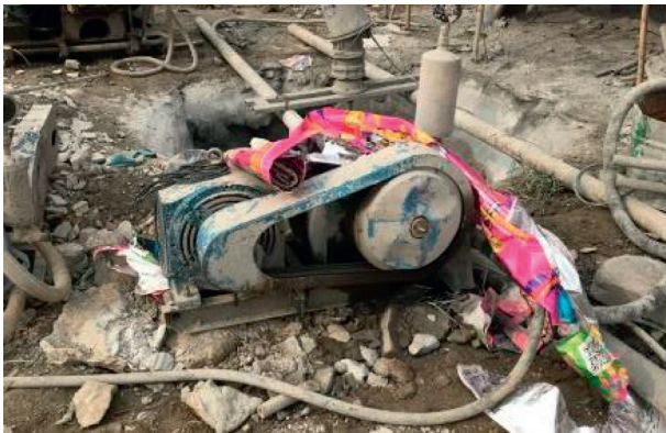
FIGURE 11: The water pump.
