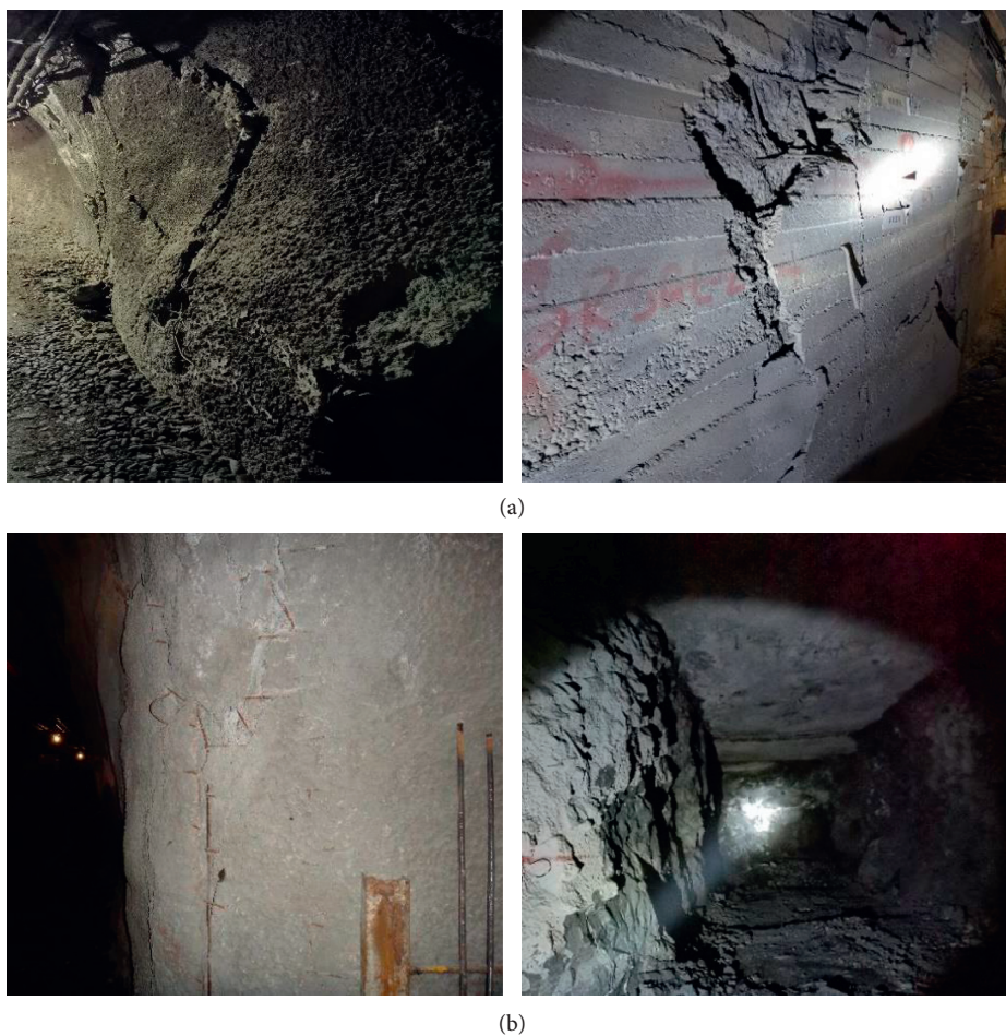
FIGURE 9: Failure patterns of the roadway (a) before and (b) after the adopted scheme IV.
