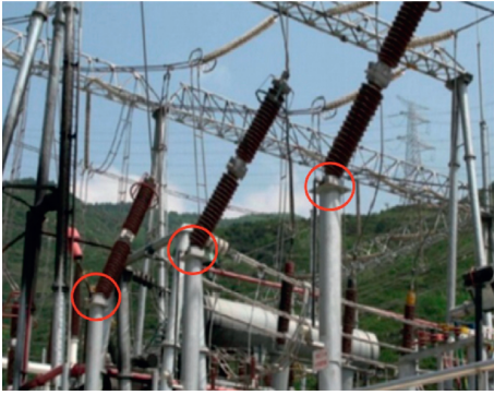
FIGURE 1: Failure of porcelain equipment after 2008 Wenchuan Earthquake [3].
