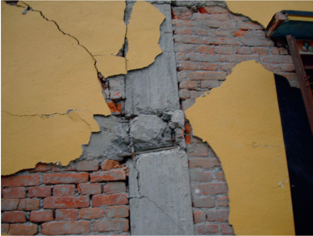
FIGURE 5: Shear damage of a column at midheight in Kathmandu due to the 2015 Gorkha earthquake.
