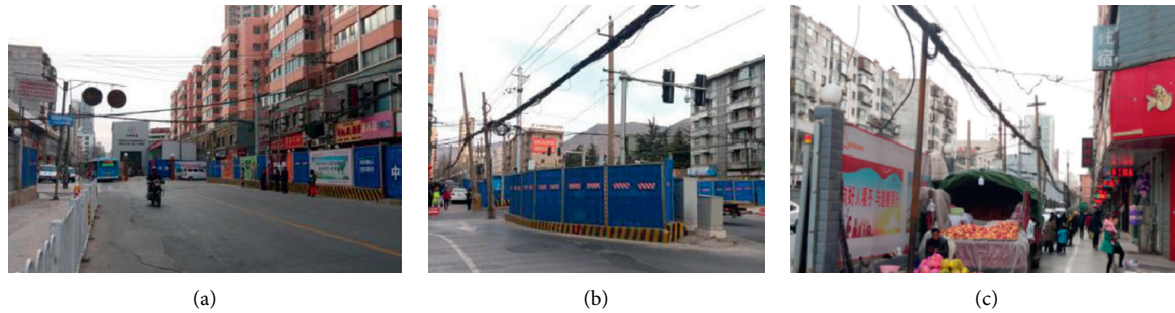
FIGURE 3: Power line status in construction section. (a) Communication lines. (b) Overhead status of communication lines. (c) Household line.
