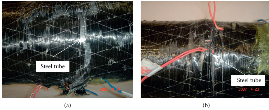
FIGURE 5: Fracture of CFRP of specimens with a small axial compression ratio. (a) Longitudinal CFRP of A1. (b) Transverse CFRP of A0.
