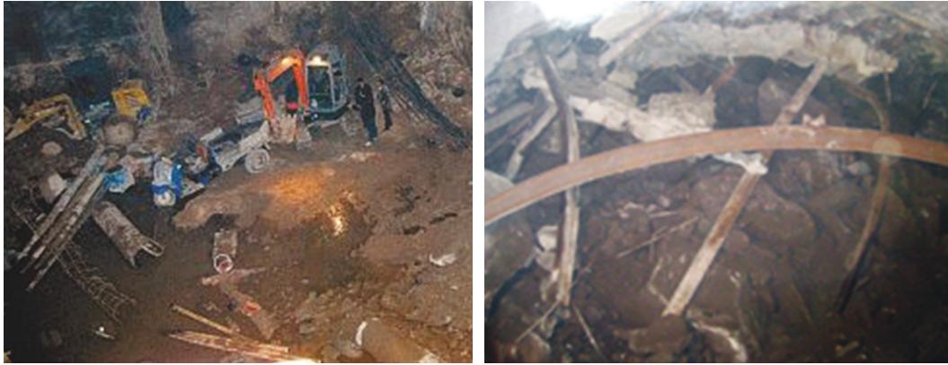
FIGURE 1: A collapse in a goaf.
