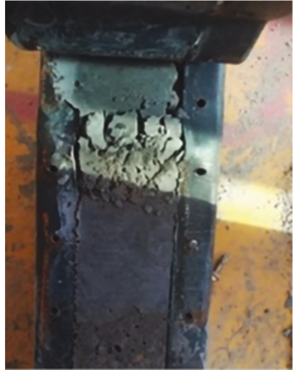
FIGURE 8: Inner concrete crushed close to the buckling wall.
