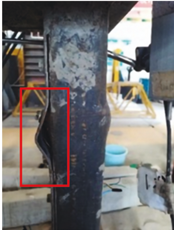
FIGURE 7: Local buckling damage.
