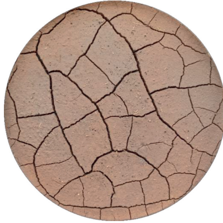
FIGURE 3: Cracks on the soil surface.
