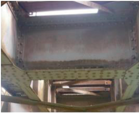
FIGURE 5: Corrosion of the deck's steel members (bottom view).
