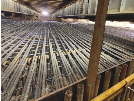
FIGURE 2: Positional relationship between horizontal steel bars in tunnel cross section and existing railway line.
