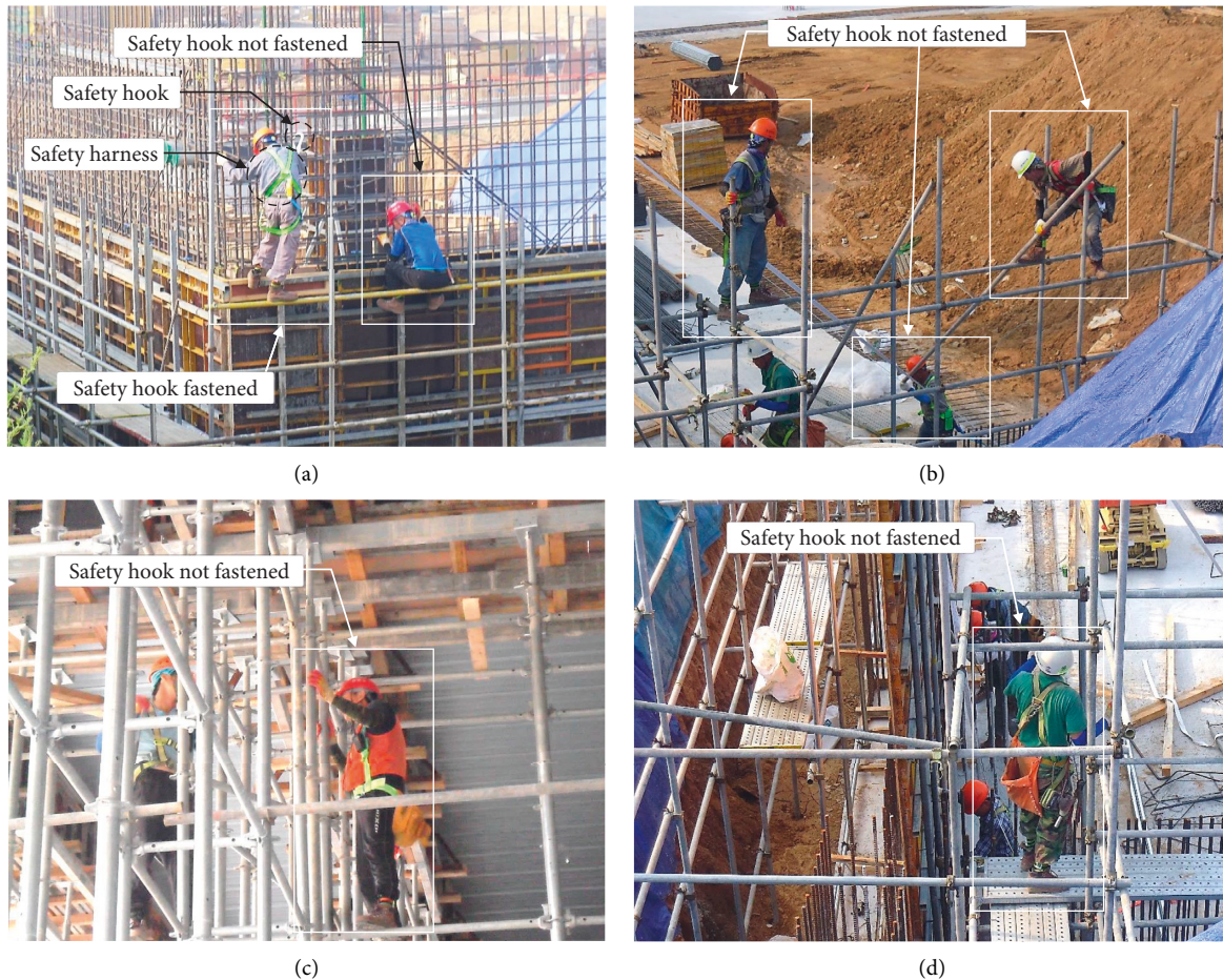
FIGURE 1: Safety harness and hook not fastened when working on the system scaffolds. (a) Formwork on the top of the scaffold. (b) Scaffold installation work. (c) Work on the Scaffoldings. (d) Moving on to the scaffold.
