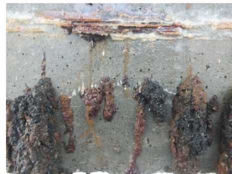
FIGURE 8: Rust products ooze out.
