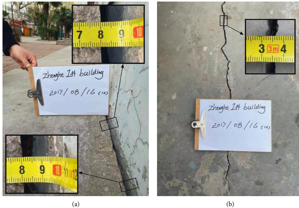
FIGURE 14: Cracks (a) between the wall and outside apron slope and (b) on the basement floor.
