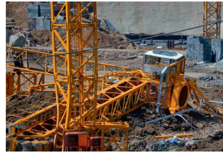
FIGURE 2: Collapsed tower crane.
