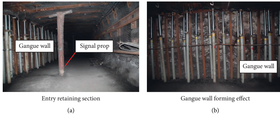
FIGURE 16: Field retaining effects. (a) Entry retaining section. (b) Gangue wall forming effect.
