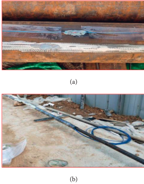
FIGURE 7: Steel pipe pile and anchor sensor installation. (a) Installation of FBG strain sensor. (b) Installation of FBG axial force sensor.
