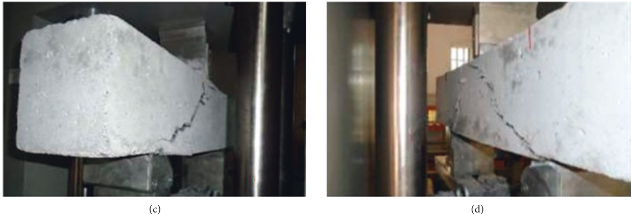
FIGURE 12: (a) Photos of failure mode of tested beams with reinforced bar, control beam, (b) photos of failure mode of tested beams with reinforced bar, at 0.25% strength beam, (c) photos of failure mode of tested beams with reinforced bar, at 0.50% strength beam, (d) photos of failure mode of tested beams with reinforced bar, at 0.75% strength beam.
