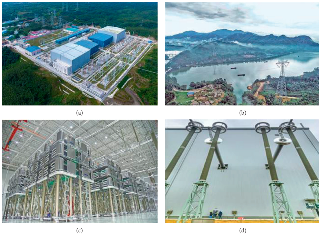
FIGURE 2: The Kunliulong DC Project construction site. (a) The \pm 800 kV converter station. (b) The Guangdong section crosses the Beijing river transmission line. (c) Construction site of VSCUHVDC converter valve. (d) Inspection site of casing through wall for VSC-HVDC.
