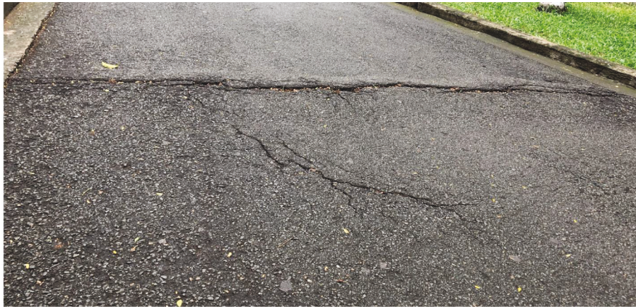
FIGURE 2: The target area including 2 cracks.
