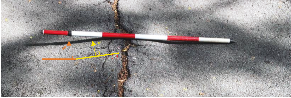
FIGURE 8: Normal vector at the crack and its neighbor area.
