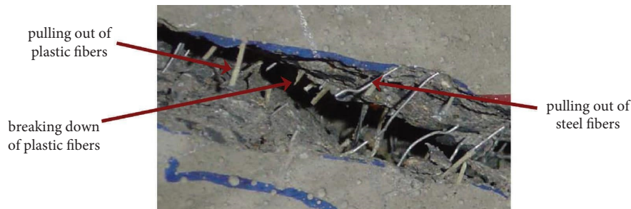
FIGURE 9: Pulling out of steel fiber and breaking down of plastic fibers in hybrid fiber-reinforced RC beam.
