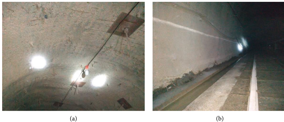
FIGURE 10: Support effect of the return-air roadway: (a) support effect of the roof and (b) support effect of the sidewall.
