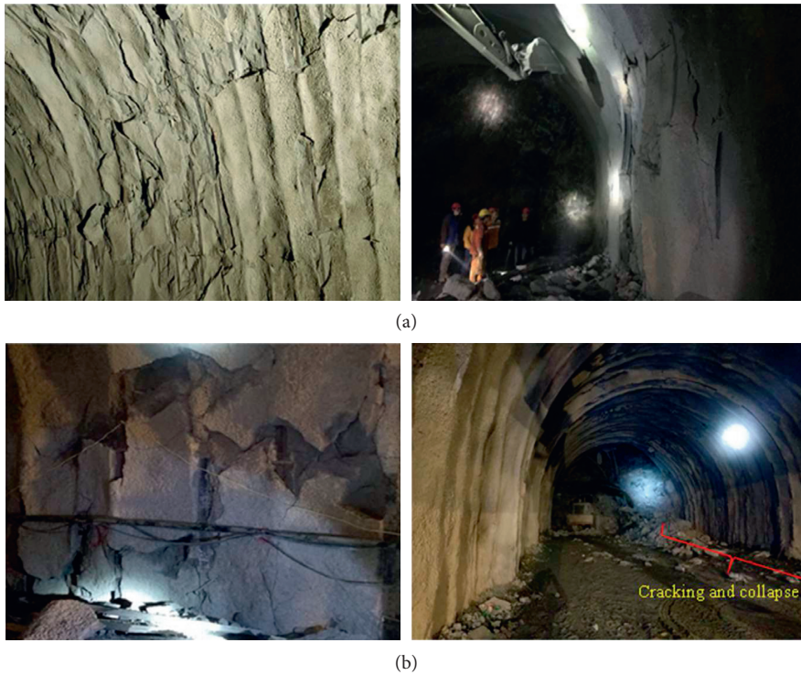
FIGURE 16: The lining crack before and after rockburst: (a) before the rockburst; and (b) after the rockburst.
