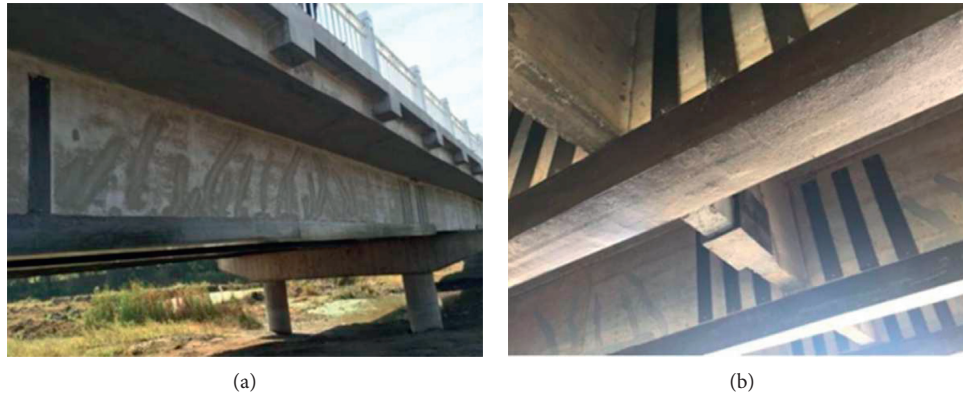
FIGURE 1: Case of solid bridge reinforcement. (a) Overall effect. (b) Beam bottom reinforcement.
