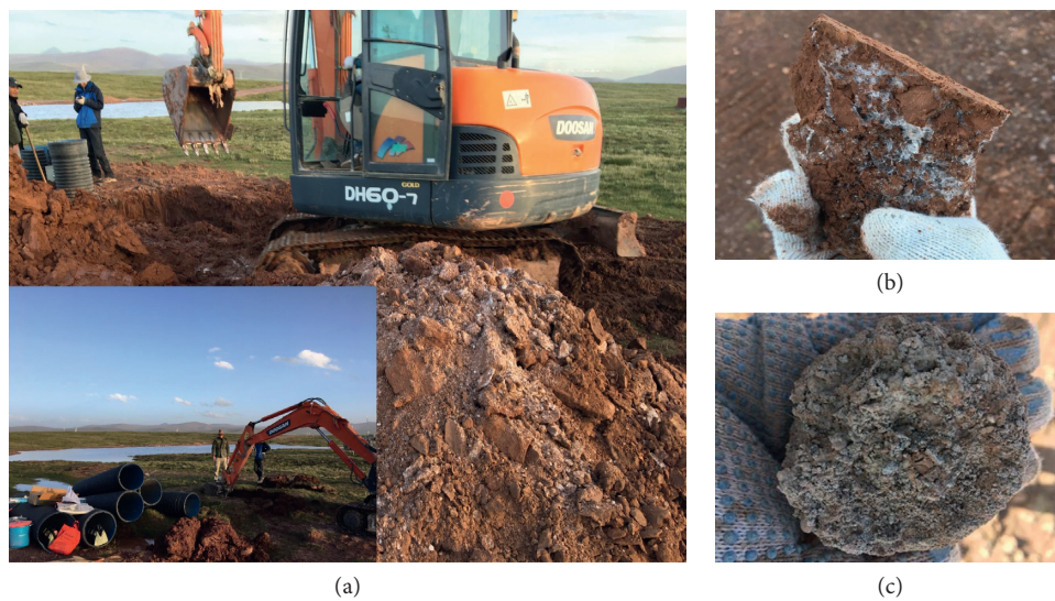
FIGURE 7: In situ test. (a) Construction site. (b) Pro-improved frozen soil. (c) Postimproved frozen soil.
