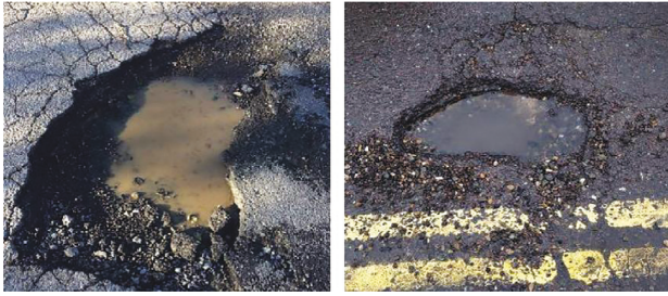
FIGURE 1: Road image having potholes [2].
