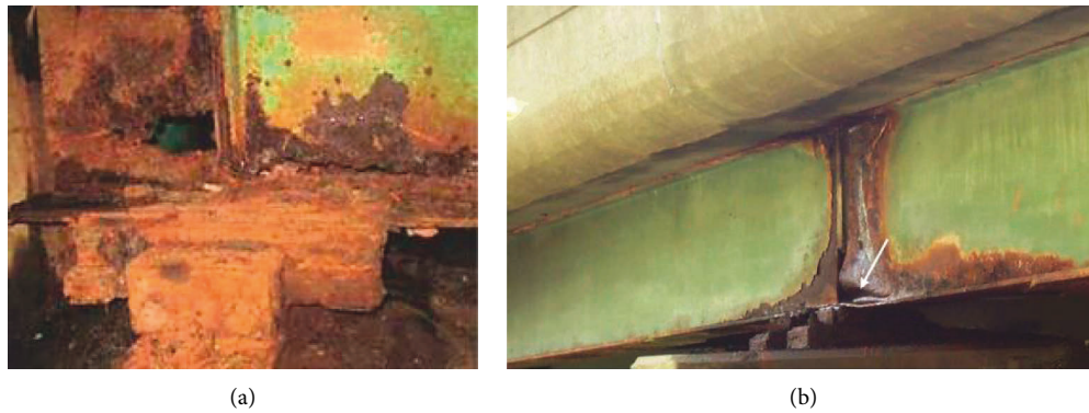
FIGURE 1: Typical corrosion damage at plate girder end: (a) Damage at bearing stiffener and web of plate girder [5], (b) corrosion damage located beneath expansion joint at the bearing [6].
