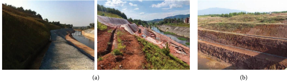
FIGURE 1: Slope in Zhetang diversion irrigation channel. (a) Danger removal of Gushan section (in 2014 and 2019); (b) typical channel section on the left bank.
