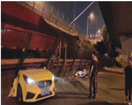
FIGURE 2: Rollover of viaduct in WuXi.
