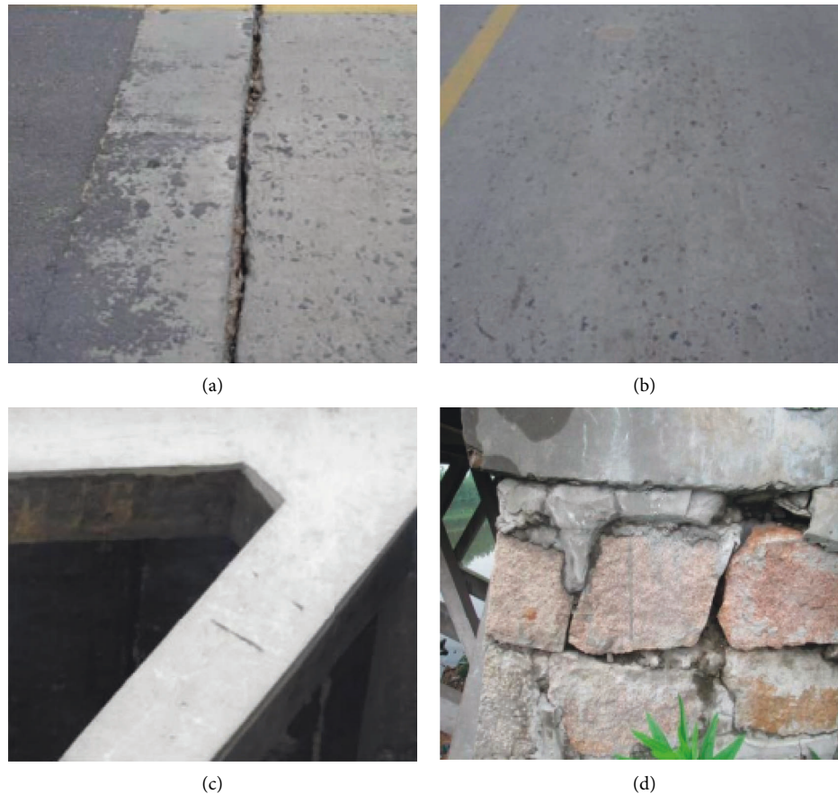
FIGURE 5: Different parts of the bridge damage. (a) Breakage expansion joint. (b) Bridge surface fracture. (c) Exposed reinforcing bar of truss beam. (d) Abutment crack.
