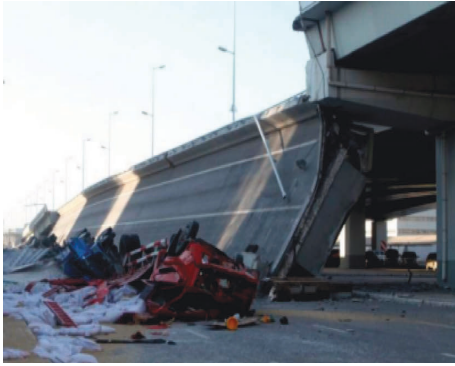
FIGURE 1: Collapse of the YangMingTan bridge.
