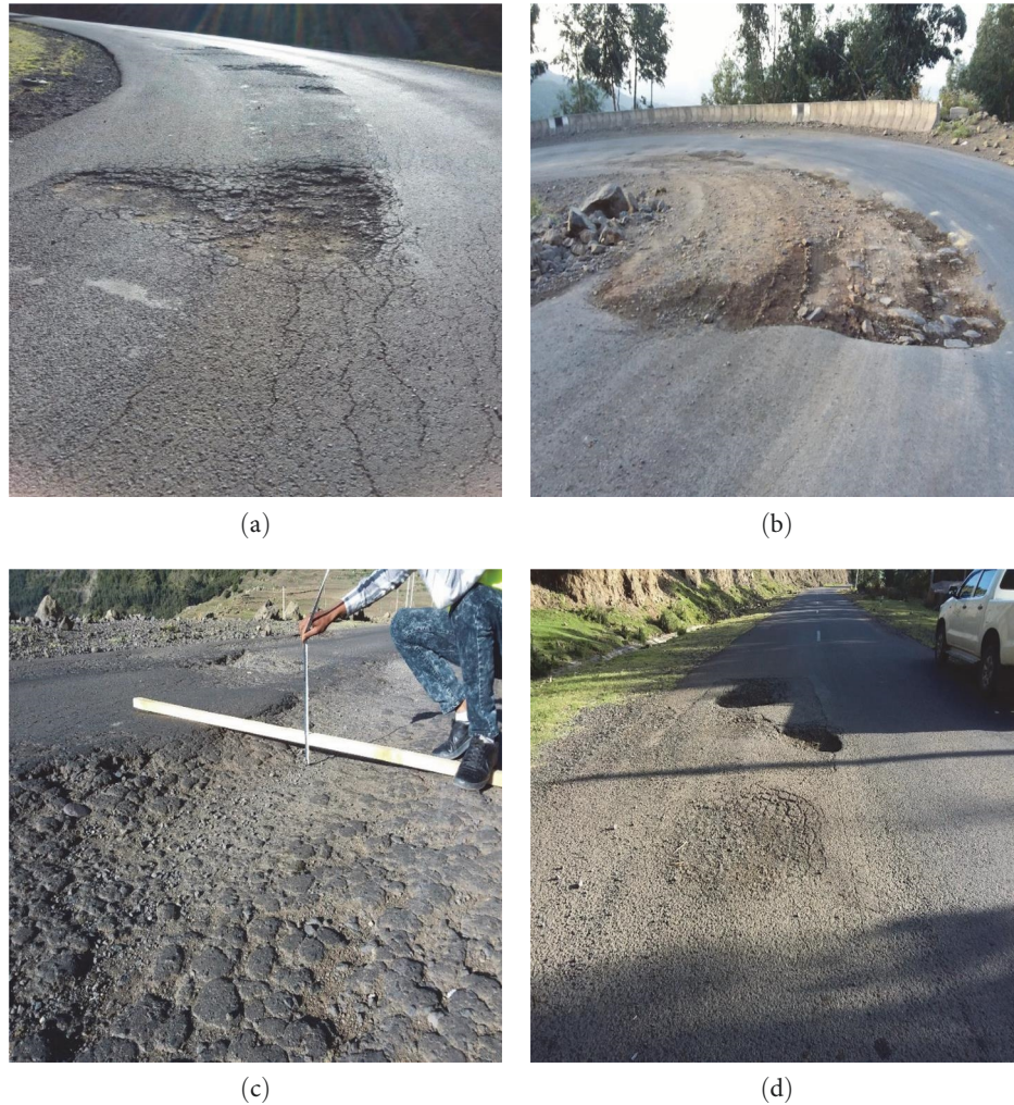
FIGURE 2: Road condition for Maichew to Adishihi asphalt road segment with (a) potholes and cracking, (b) pavement deformation at a curve, (c) rutting and raveling, and (d) patches with pothole defects.
