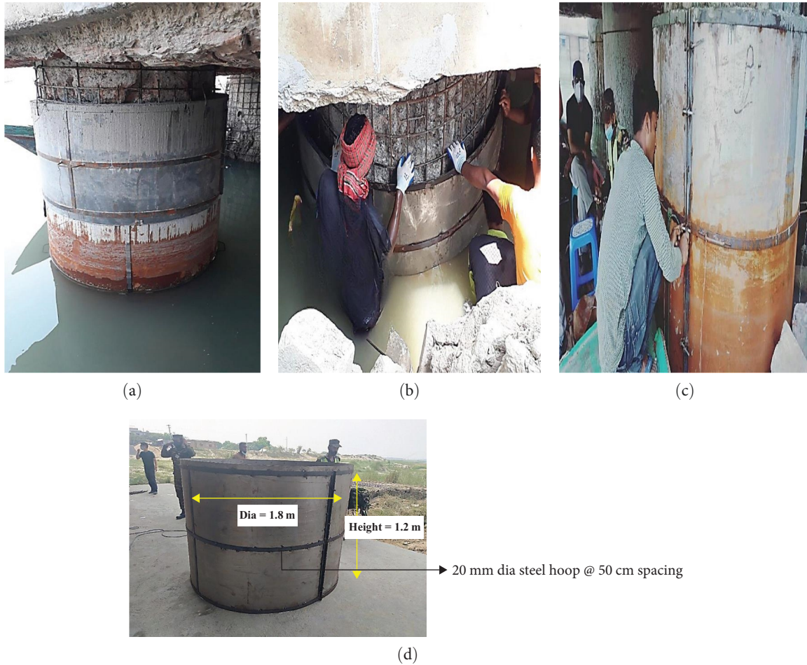
FIGURE 18: (a)–(c) Placement of permanent casing process and (d) iron permanent casing dimension.
