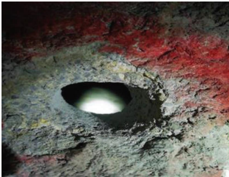
FIGURE 13: Void behind the lining.
