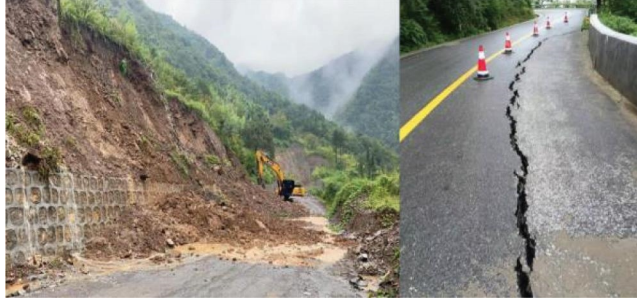
FIGURE 1: Cutting slope slip and subgrade cracks.
