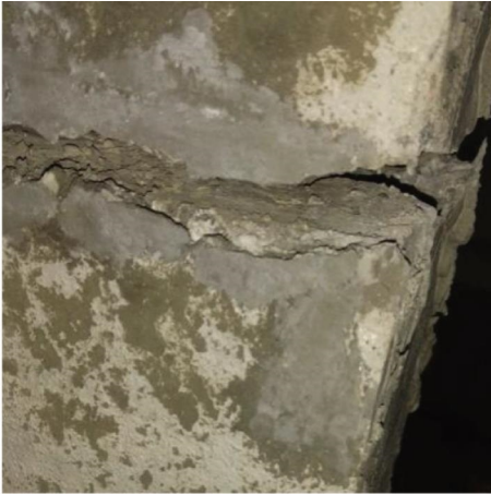
FIGURE 21: Precast wall panel—slender 2—failure.
