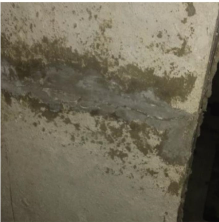
FIGURE 22: Precast wall panel—intermediate 1—failure.
