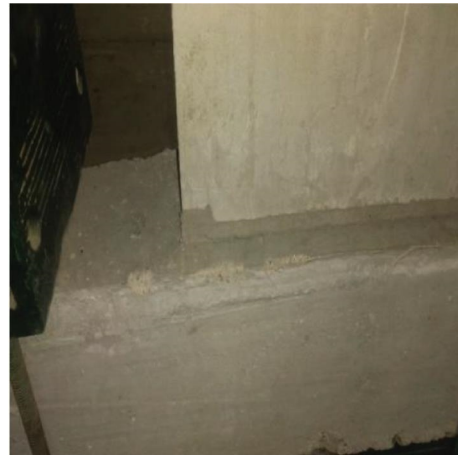
FIGURE 19: Monolithic wall panel—intermediate—failure.
