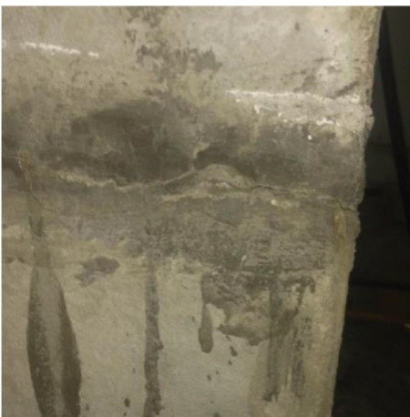
FIGURE 23: Precast wall panel—intermediate 2—failure.
