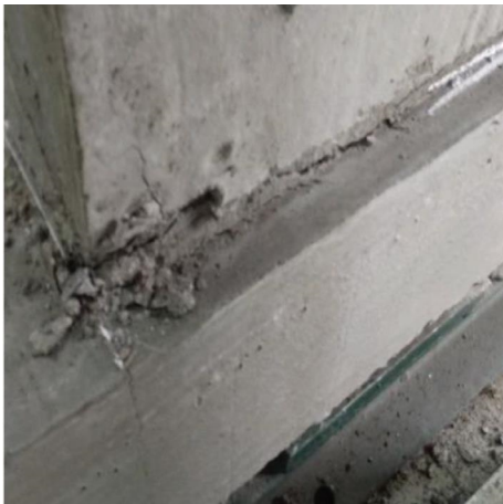
FIGURE 18: Monolithic wall panel—slender—failure.
