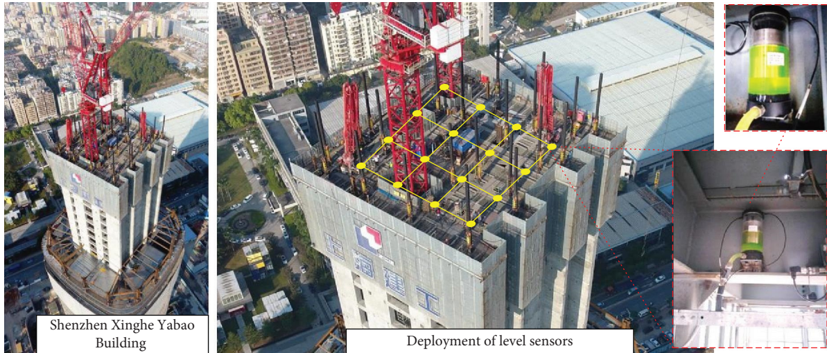
FIGURE 7: Deployment of level sensors for the HBM in the Shenzhen Xinghe Yabao Building.
