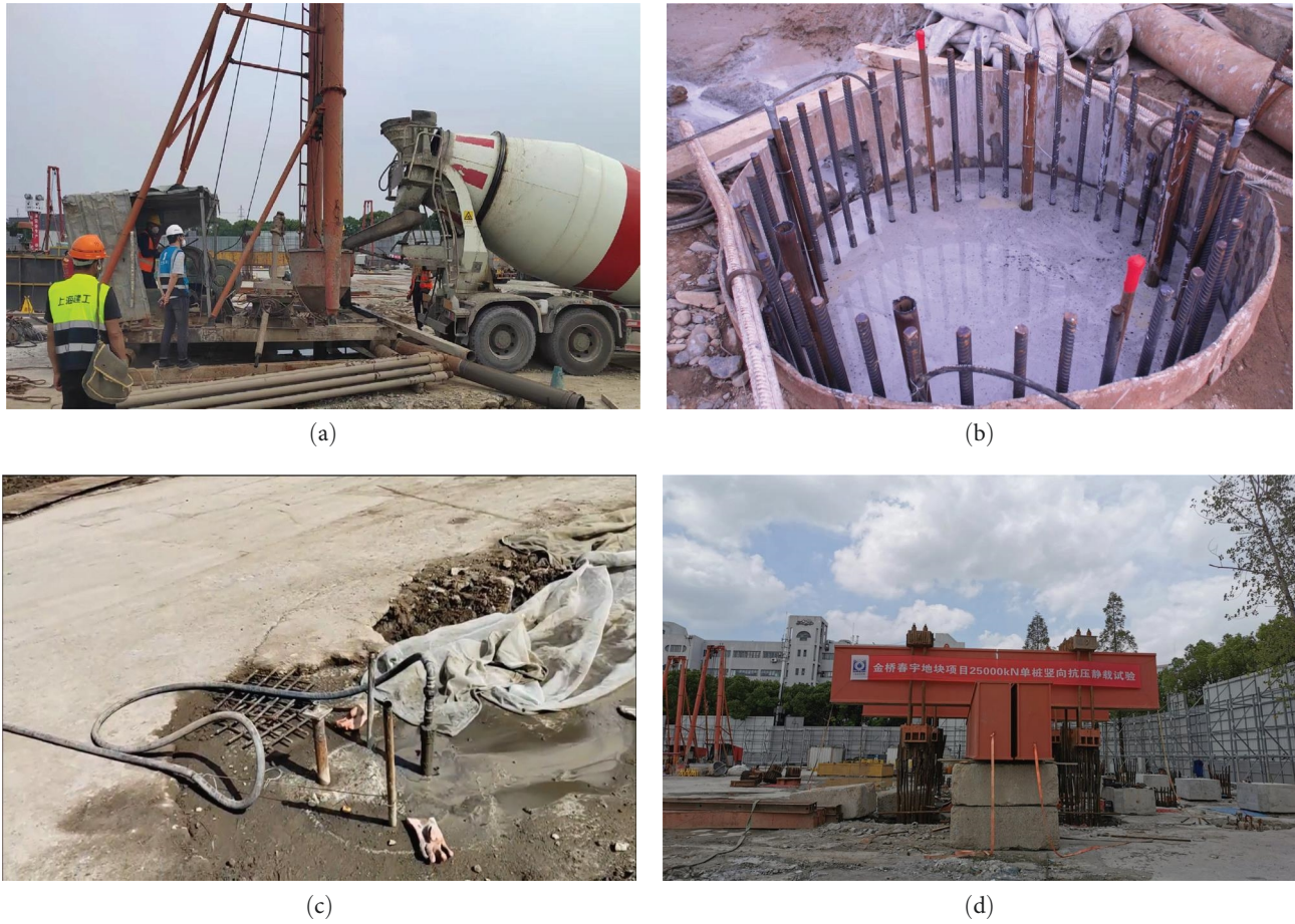
FIGURE 4: Photos of the field trials at the Jinqiao-Chunyu site: (a) construction of a cast-in-place pile; (b) head of a cast-in-place pile; (c) postgrouting; and (d) static loading test.
