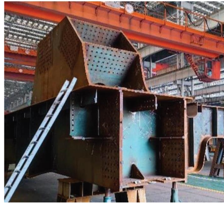
FIGURE 17: Site view of the lower chord bar.
