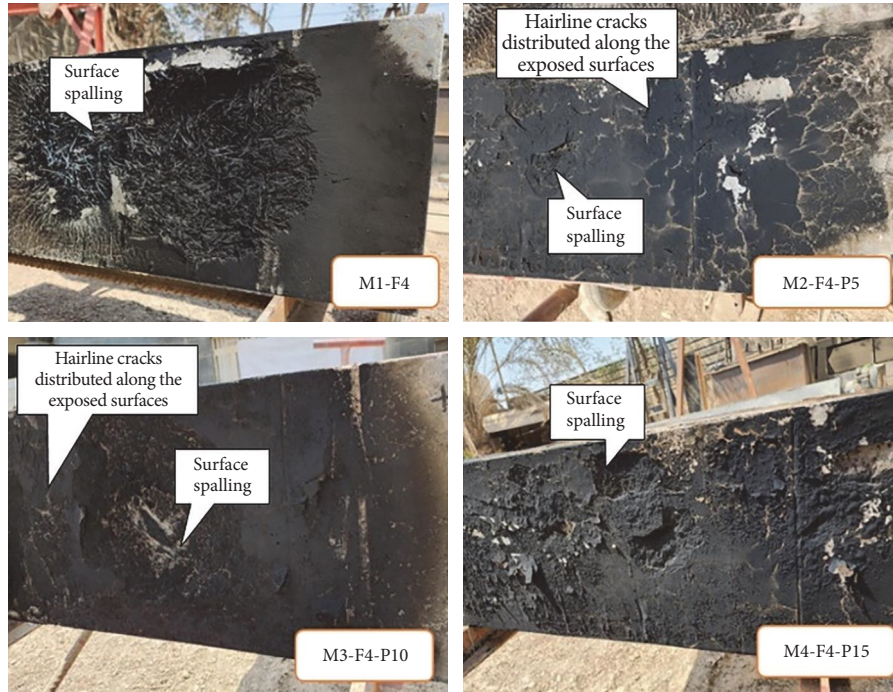
FIGURE 16: Photos of SIFCON specimen surface after exposure to a fire flame at 600°C.
