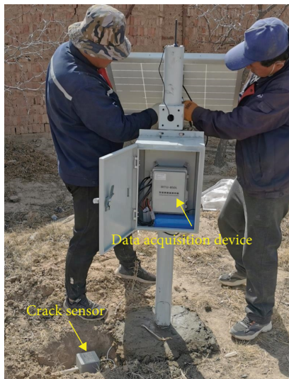
FIGURE 8: Monitoring equipment for landslide deformation.
