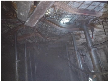
FIGURE 6: Deformation of the roof of the roadway.
