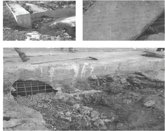
FIGURE 1: The deterioration of concrete examples from the locations.
