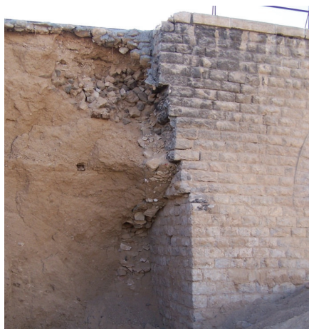
FIGURE 4: Abutment failure that shows the fill materials.
