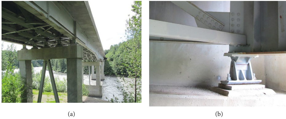
FIGURE 1: Photographs of the bridge system: (a) Chulitna River Bridge and (b) expansion bearing condition.
