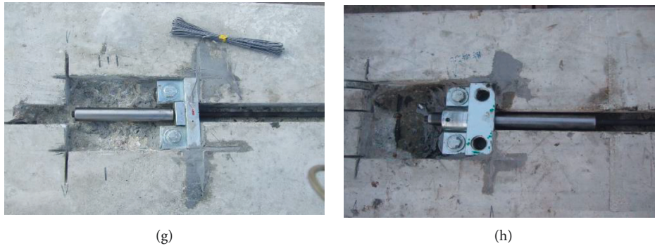
FIGURE 13: Installation process of anchor and FRP tendon. (a) Grooving. (b) Drilling of anchor bolt holes. (c) Leveling of groove by epoxy. (d) Fastening of anchor bolt. (e) Installation of anchor bolt using torque wrench. (f) Installed anchor. (g) Fixation of anchor at the fixed end by washer. (h) Nut fastening of anchor in jacking end.
