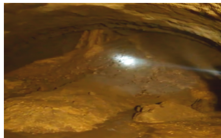
FIGURE 6: Site of tunnel collapse sand.
