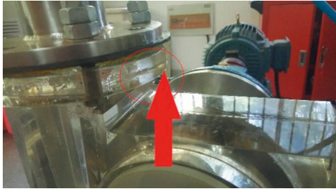
FIGURE 23: Location of pump shell crack.
